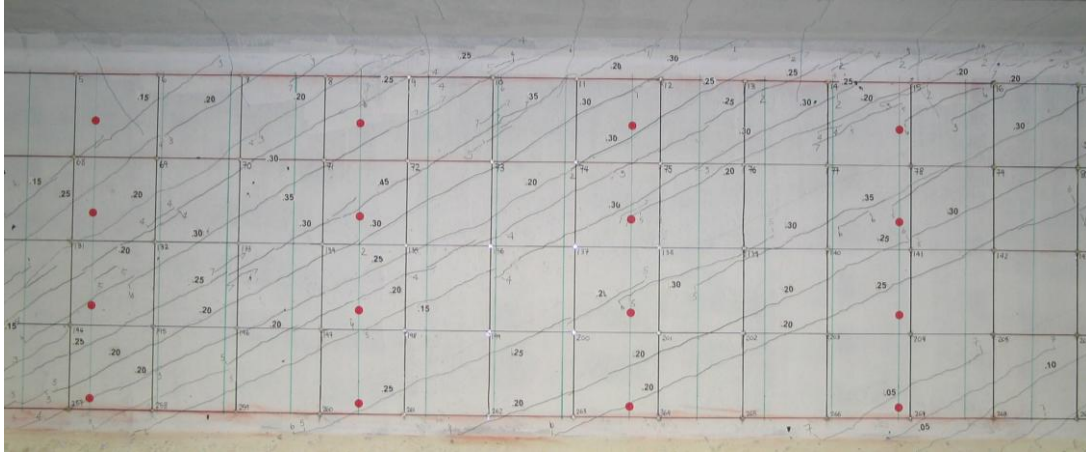
Fig. 10.7: Cracking patterns which demonstrate that beam shear behaviour was achieved
