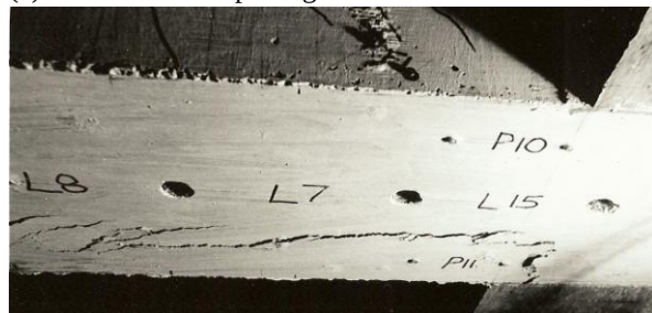
(b) View of cover spalling from below
