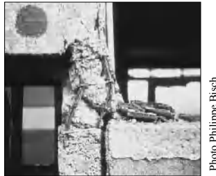
Figure 9.4. Rupture of a column due to the shock between two neighboring structures
