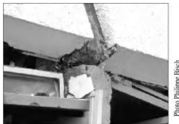
Figure 9.5. Rupture of a section due to insufficient longitudinal reinforcements
