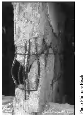
Figure 9.12. Rupture of a column due to buckling of longitudinal reinforcement
